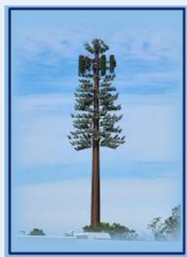
Faux California Pine Wireless Installation
